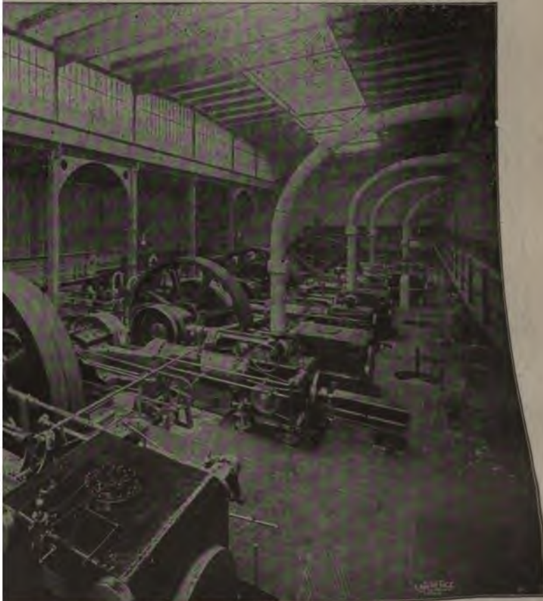
OR OF A CABLE-RAILWAY POWER-HOUSE. passing over the wheels which move and stretch them.
